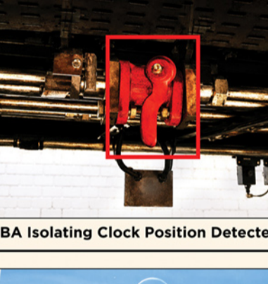
Stay Rod Broken Detected
